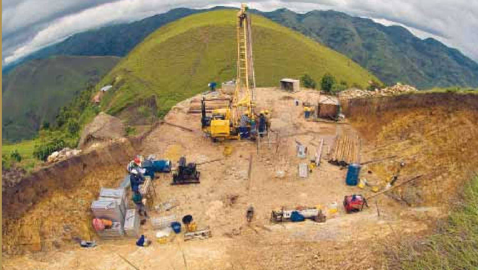
A diamond drill rig belonging to South Africa's Geosearch working at the Twangiza project.
